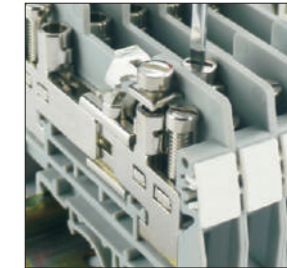
Figure 1, switching jumper: for two terminal blocks, usable for both sides of the disconnect slide.
